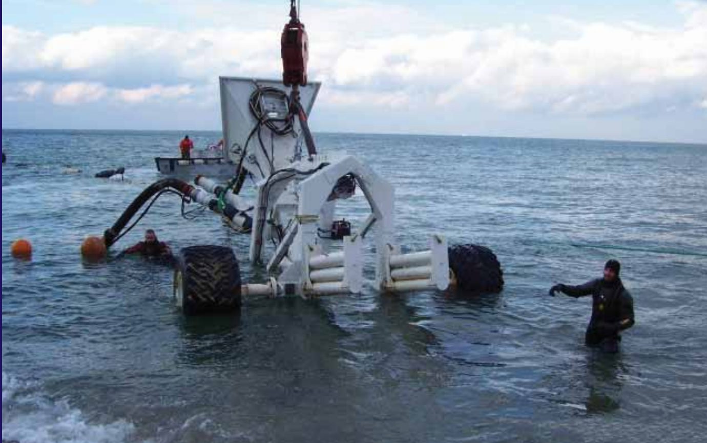
As the plow travels along the seabed, it liquefies the soil ahead of the plow using water jets on the plow blade. The cable passes through the hollow plow blade and is buried approximately 6 feet below the seabed. The temporarily liquefied area almost immediately fills back in as the sediment naturally resettles.
