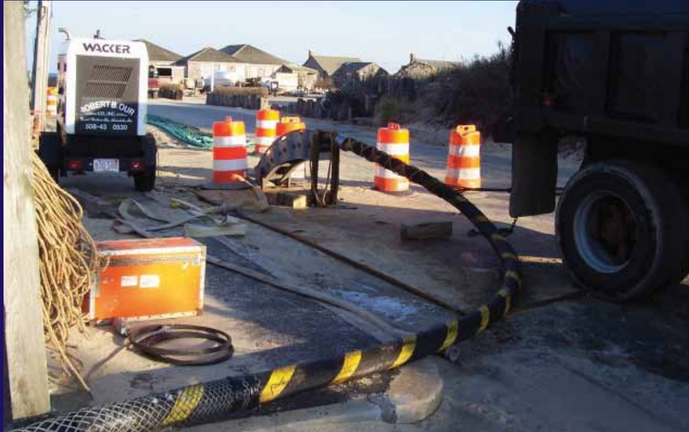
Once the submarine cable is laid, it is then connected to an underground cable inside a manhole near the shore.
