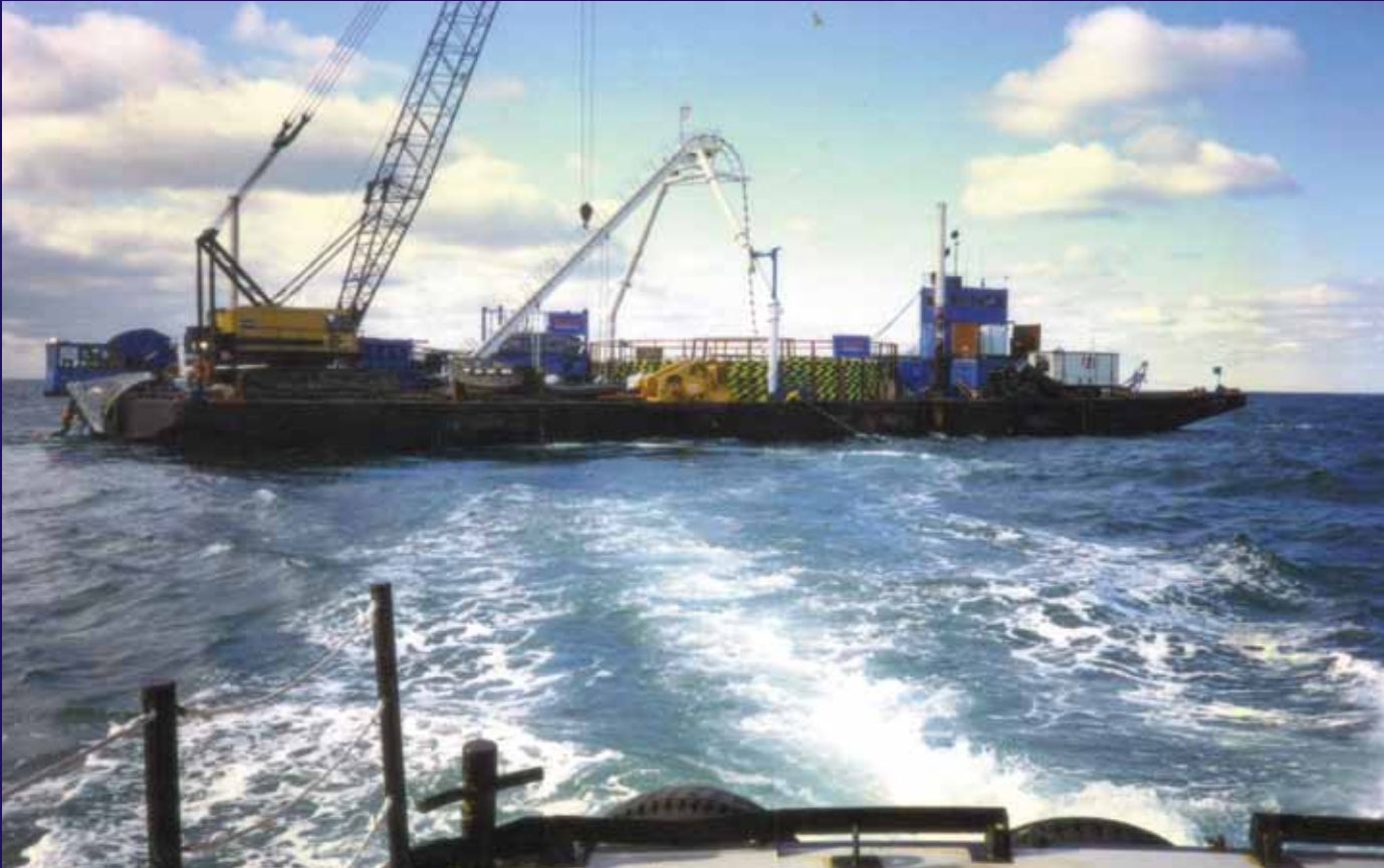
The cable is fed through the plow from a vessel similar to the one pictured above.
